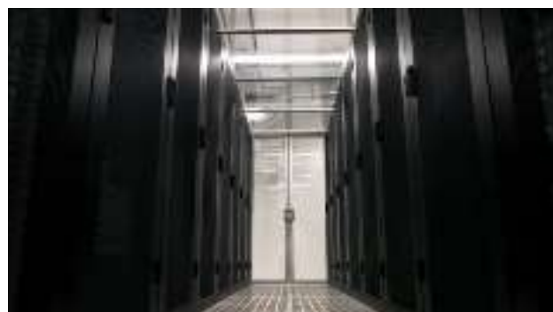
▶ Small-scale server room
