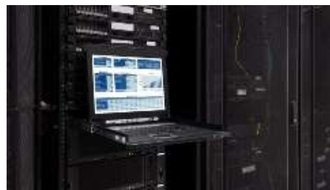
◀ Communication base station
